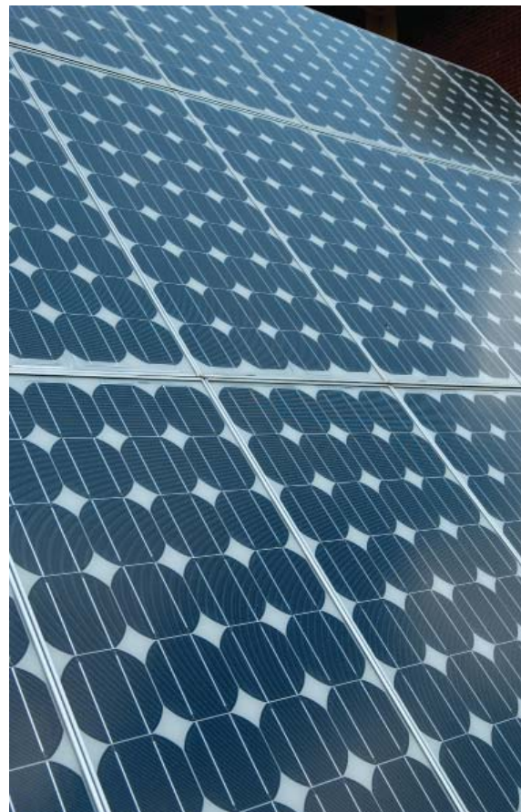
Fig.: Photovoltaic modules made of crystalline silicon
