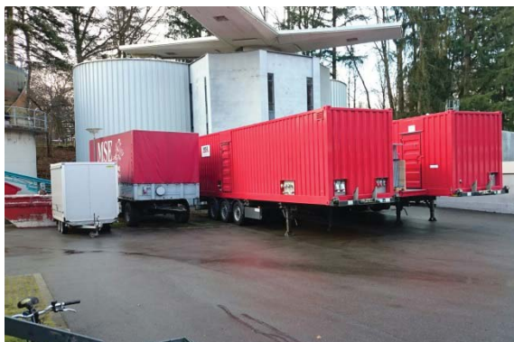
Figure 1: Mobile Phosphorus recovery plant
