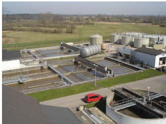
Figure: Primary clarification, combined heat and power plant, and biogas plant of the wastewater treatment plant in Baden-Baden
