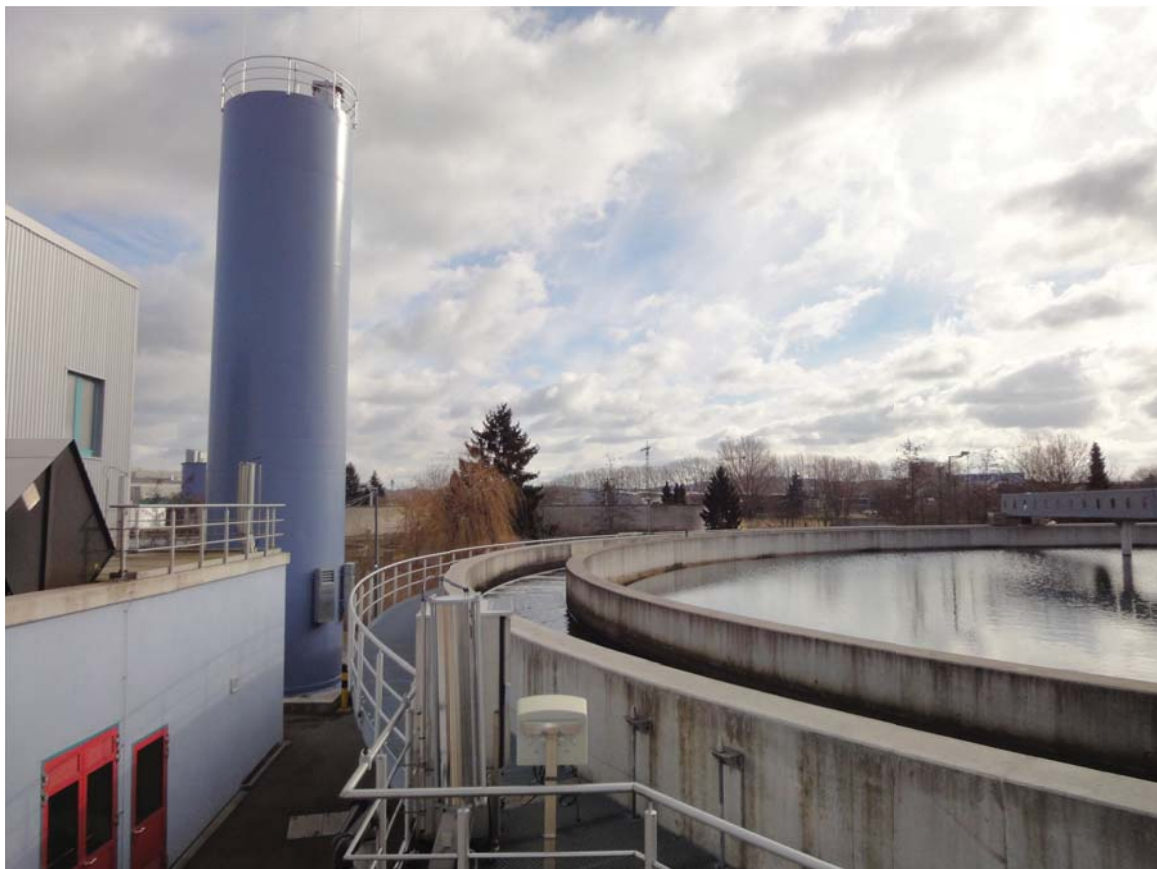
Figure 1: Further purification stage using powdered activated carbon for targeted elimination of trace substances at the Böblingen-Sindelfingen wastewater treatment plant (Source: KomS)
