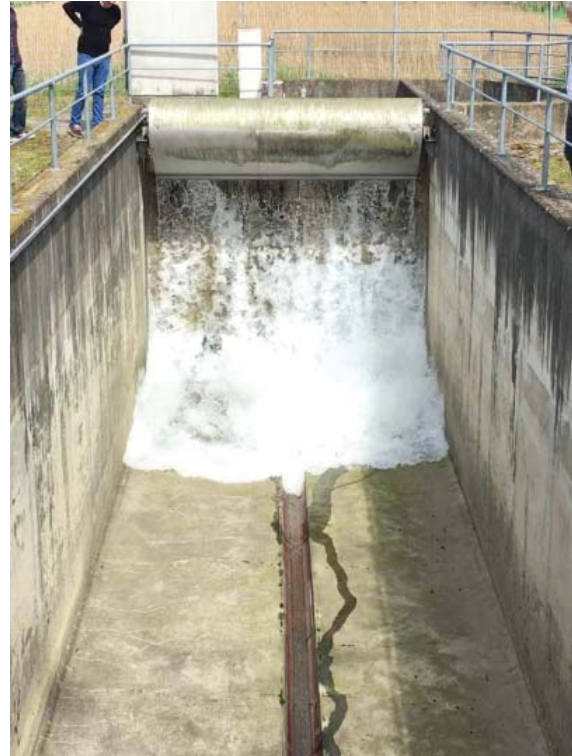
Figure: Tipping bucket flushing a CSO tank
