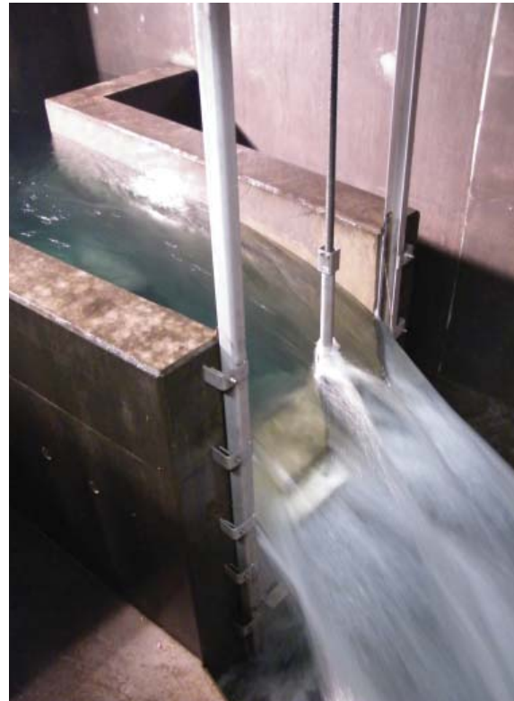
Figure: Clear water discharge after sedimentation process
